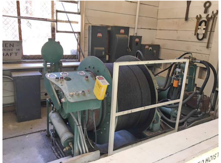
Lawry Shaft Hoist
